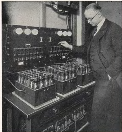
A typical Willard installation in a broadcasting station
