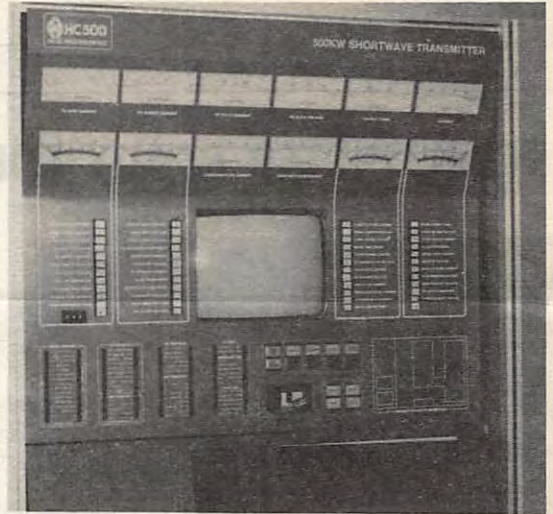
500-kW transmitter control panel
