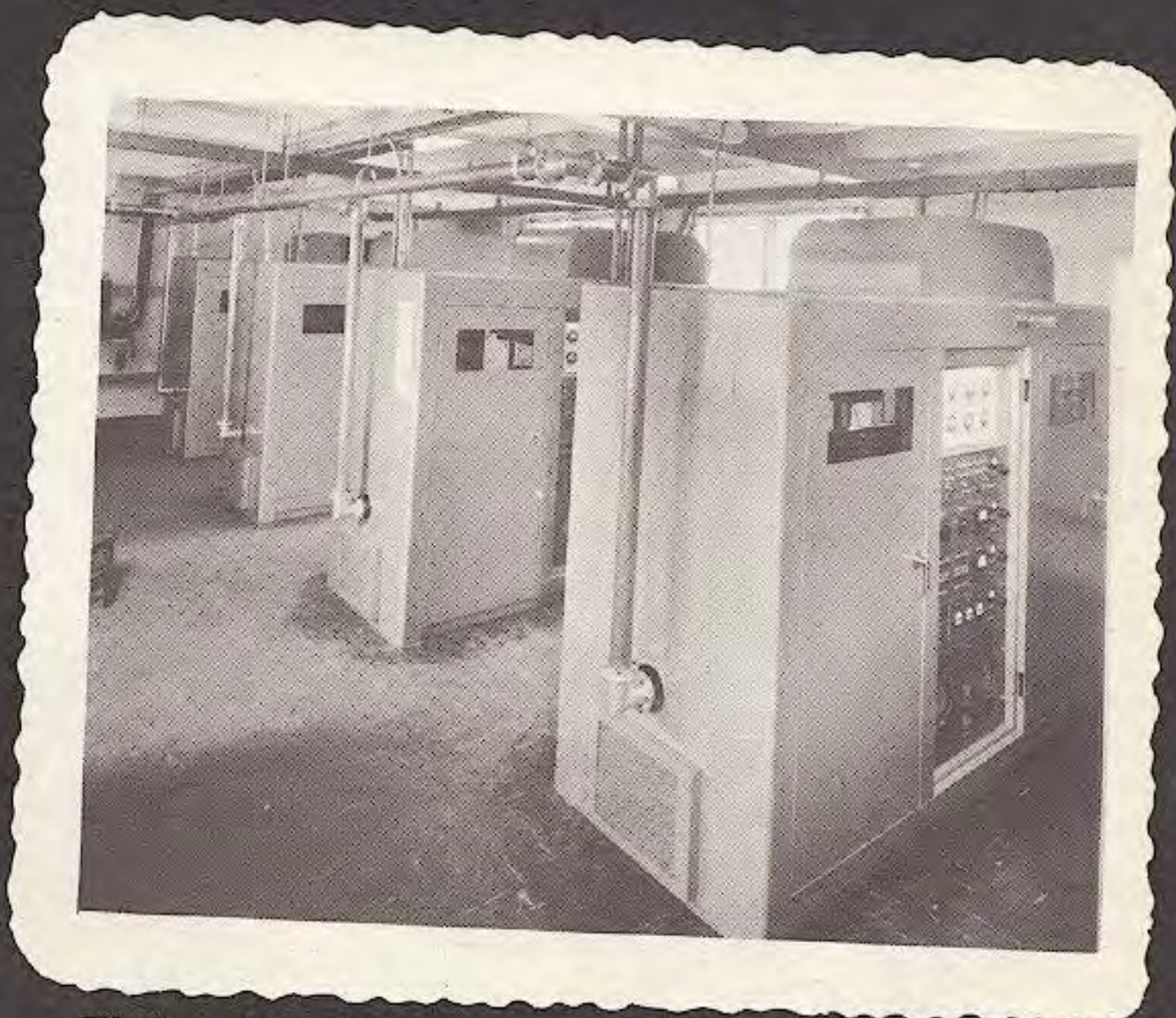
This 50 KW transmitter is part of NATO's main communications trunk -- the "Ace High" tropo system.
