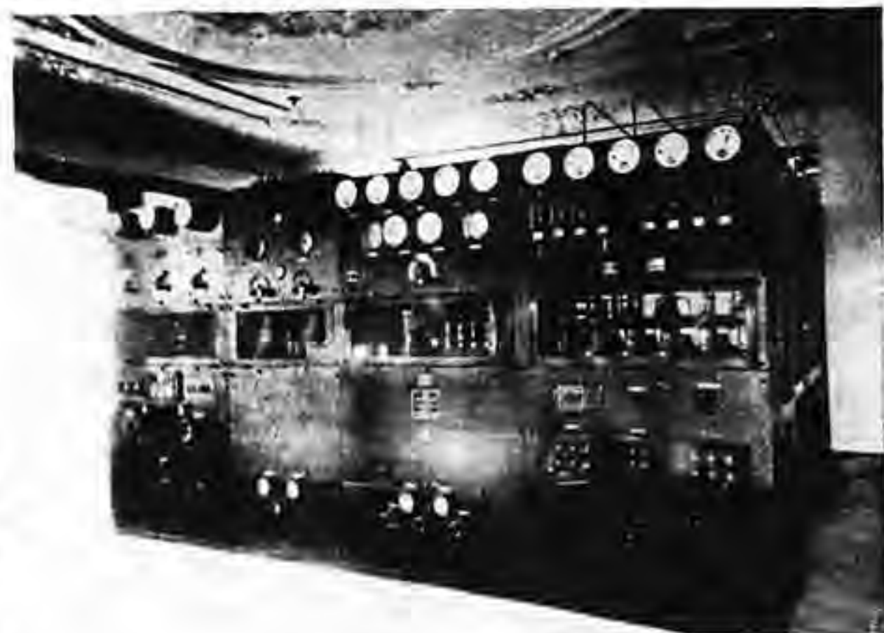
Transmitter and control panels at station XEB, Mexico City.
