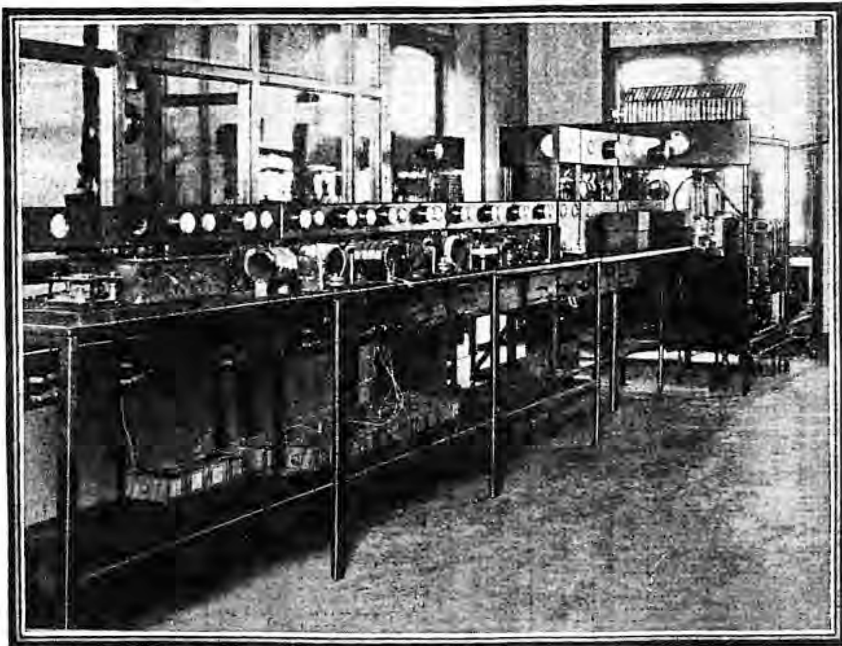
The short-wave transmitters of KDKA are housed in the same building with the long-wave sender. Above is shown some of the short-wave equipment, with a transmitter at the rear.
