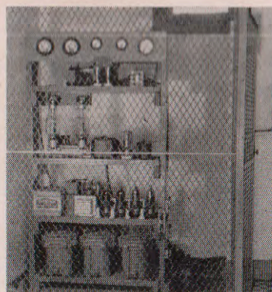
• Power Supply and Modulator Unit of W9XA
