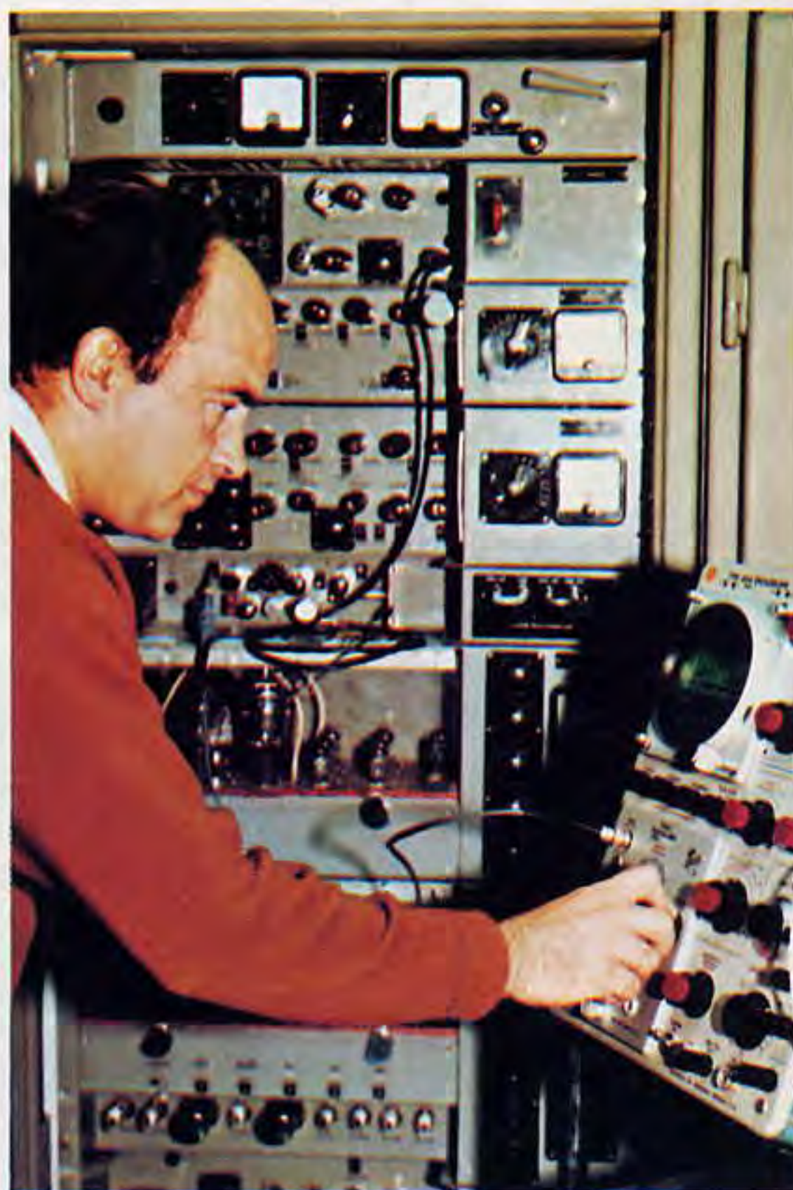
Technician at Mount Dandenong transmitter adjusting an oscilloscope to ensure that frequency modulation is functioning correctly.
