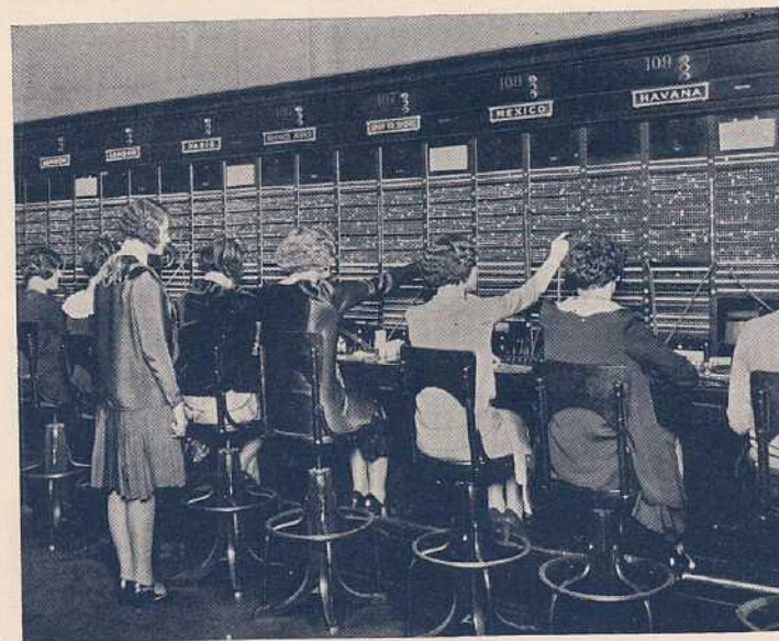
Switchboard at New York Long Distance office, where all Overseas Calls are handled
