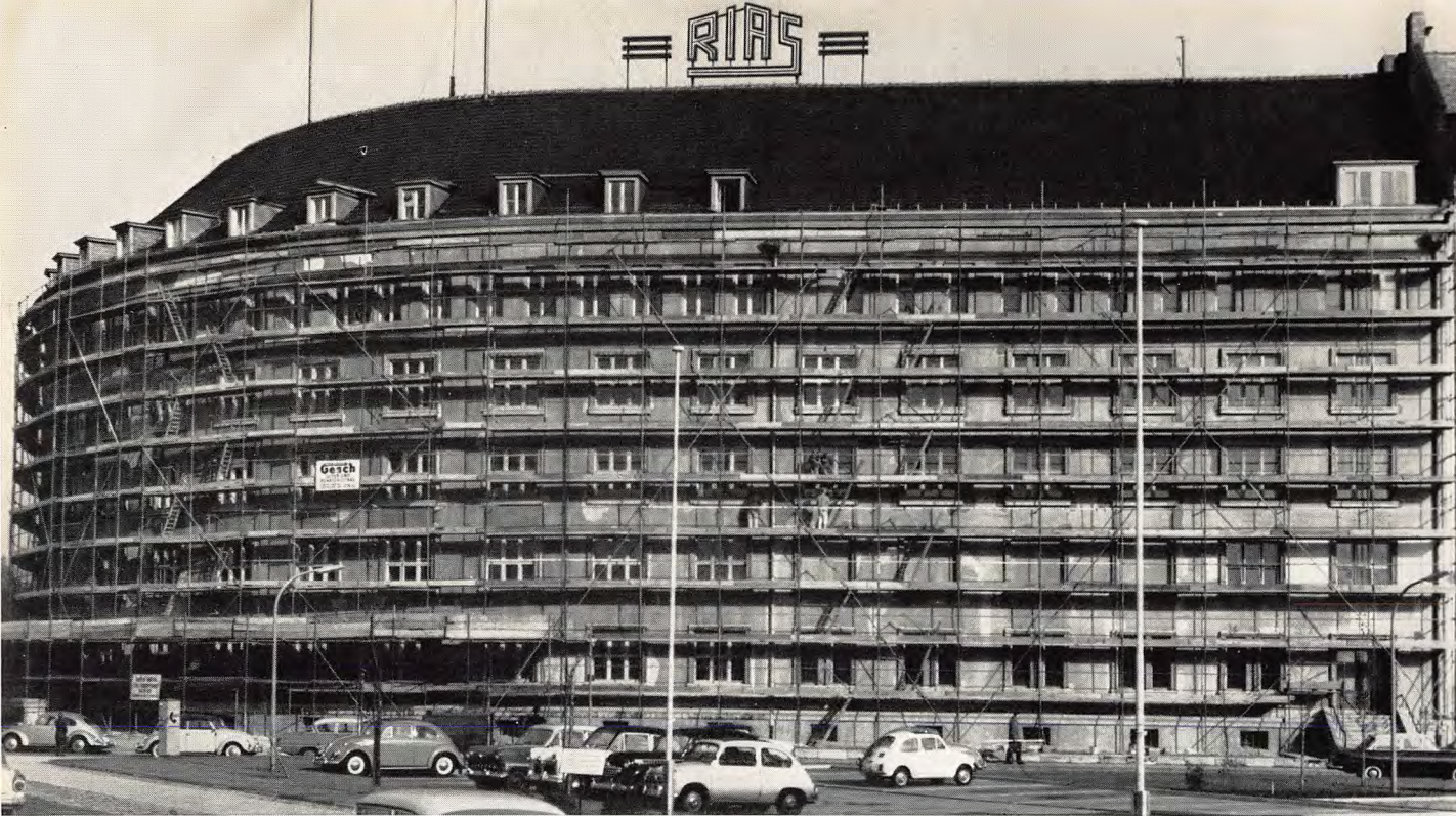
▲ In the fall of 1961, the façade of the RIAS studio building was repaired and painted
