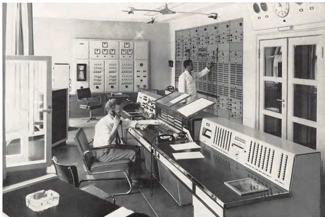
▲ RIAS Master Control regulates program output to the entire battery of transmitters in Berlin, as well as output to the long distance telephone lines carrying the program to Hof and Munich
