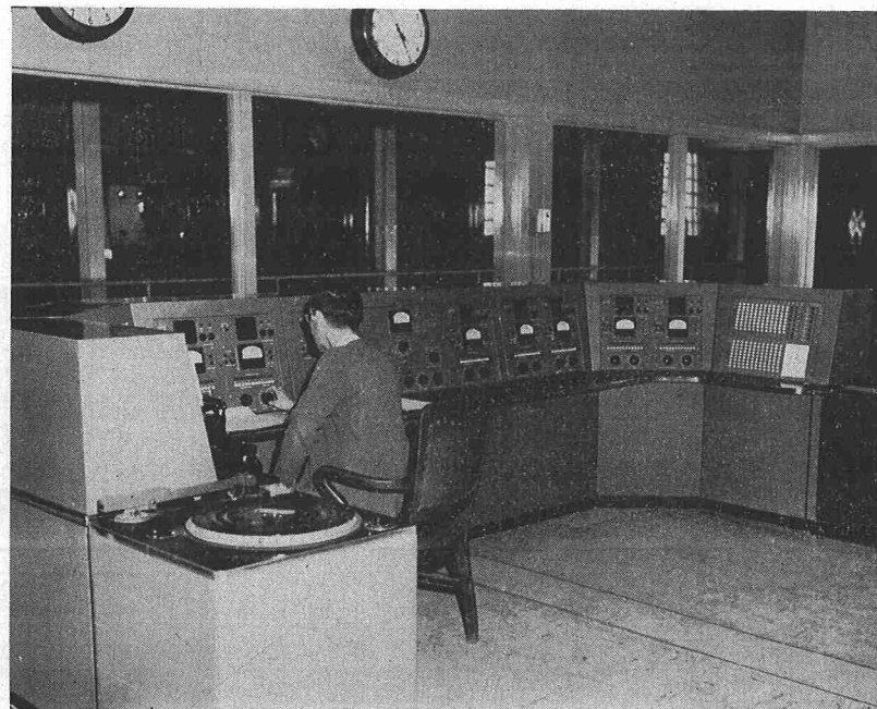
Figure 4—Transmitter control room with master control console in an overseas relay station.
