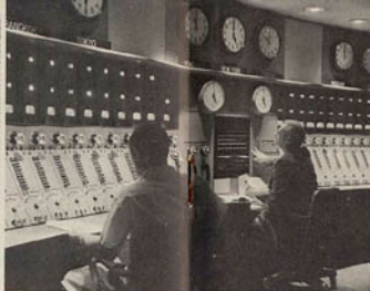
Two technicians are on duty around the clock at Master Control Board, which can feed 26 programs to Voice's U.S. transmitters at the same time and can switch all channels at every station break.
