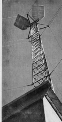
Greenville end of microwave.
